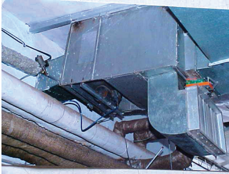
Fig. 8.15. Modified AHU with fresh air fans
