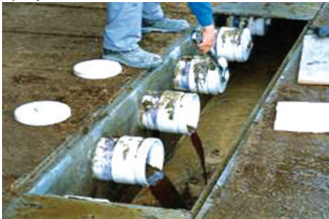
Fig. 7.11. Under stack aeration ducts
