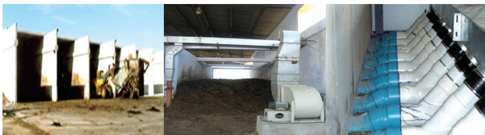
Fig. 7.18. Bunkers and ventilation systems
