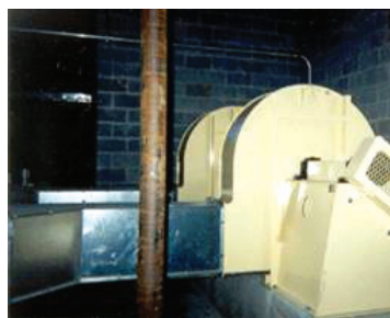
Fig. 8.10. Tunnel with air handling unit
